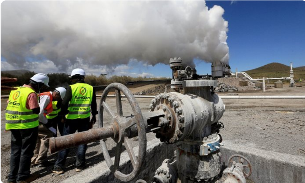
Kenya Electricity Generating Company (KenGen) workers are seen at a section of the Olkaria IV geothermal power plant near the Rift Valley town of Naivasha, Kenya. 2018. Reuters/Thomas Mukoya
